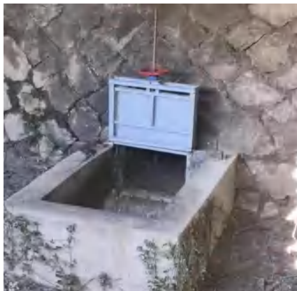
污水处理二站雨水口水闸
